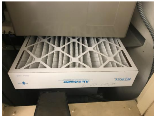
Typical Gas Fired Furnace Closet & MERV-13 Fresh Filter
