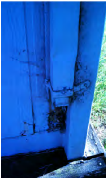
DAMAGED RAIN LEADER AND SURROUNDING FINISH MATERIALS
