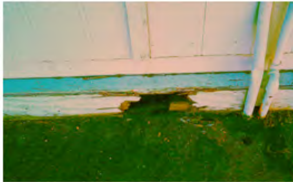
TYPICAL BUILDING FLOOR SILL PLATE IN CONTACT WITH GRADE. THIS WAS OBSERVED PRIMARILY AT THE EAST ENDS OF BUILDINGS A,B AND ADMIN
