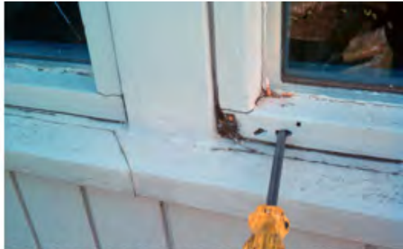
DRY ROT TYPICAL AT EXPOSED WINDOW FRAMES
