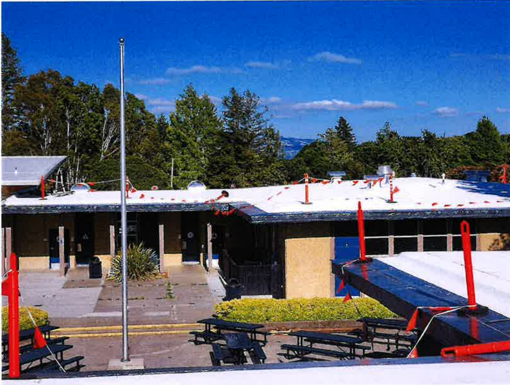
Roof view looking towards Building B as of 7/7/22 with Reflective cap sheet.
