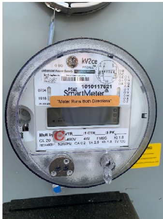
PG&E Electric Meter
