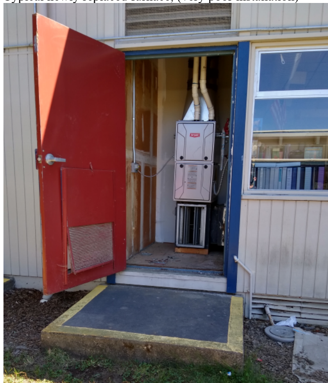
Typical newly replaced furnace, (very poor installation)
