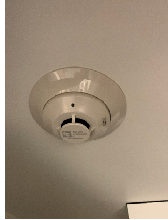
Typical Smoke Detector
