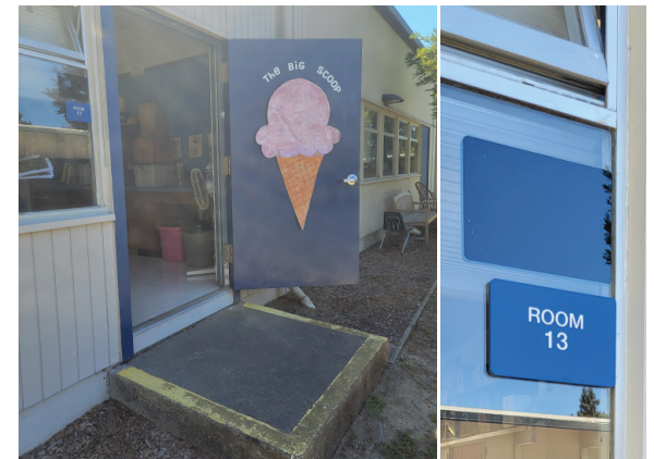
Classroom exterior non compliant doors/signage
