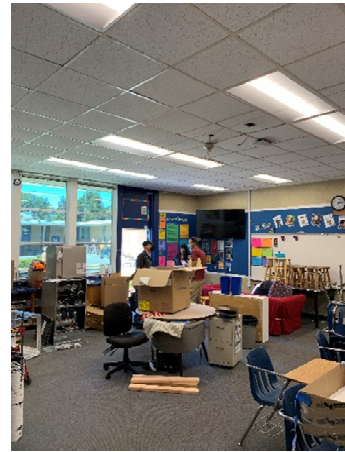
Recessed Classroom Ltg
