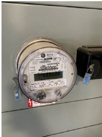
PG&E Electric Meter
