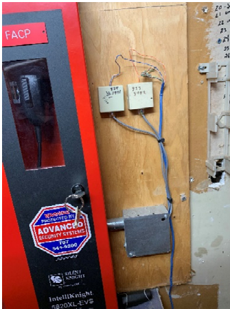
Off-Site Monitoring Lines
