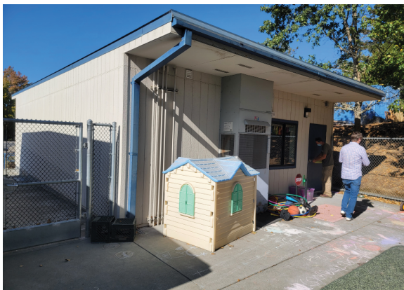
Exterior Building J - moisture intrusion at soffit
