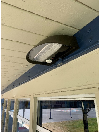
Exterior LED Lighting
