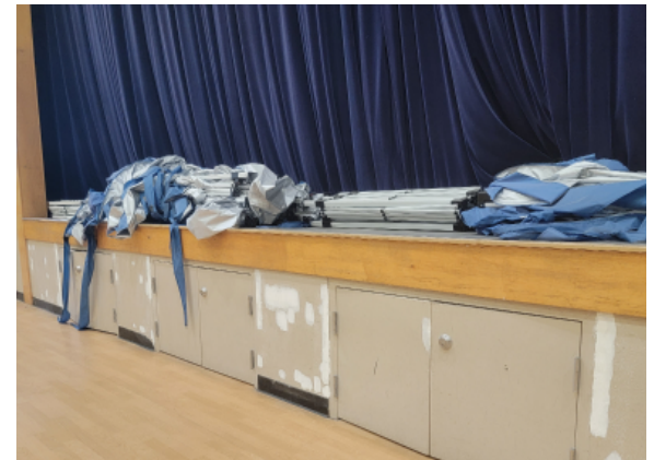
Area beneath stage in need of repair.
