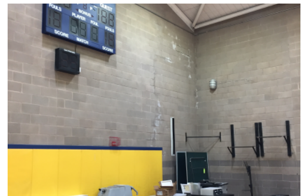
MPR Interior - Efflorescence at CMU
