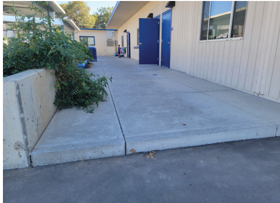
Non-accessible path at Building G to playground
