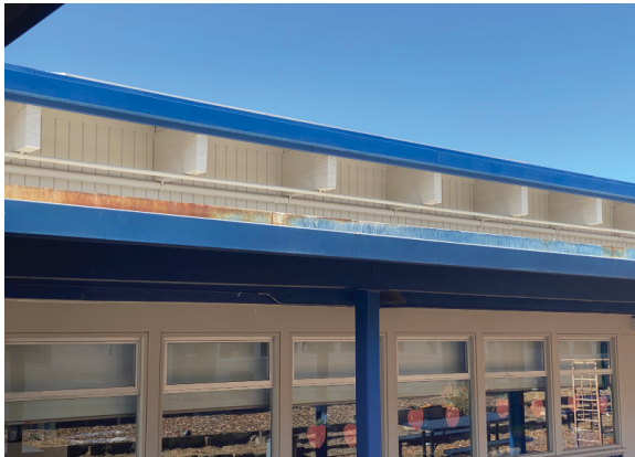
Corrosion at mechanical vents (exterior)
