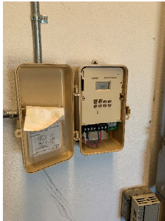
Exterior Lighting Timeclock
