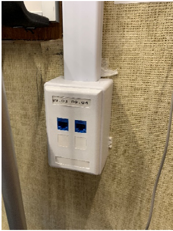
Hard Wired Data Jacks
