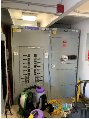
Main Electric Service Panel
