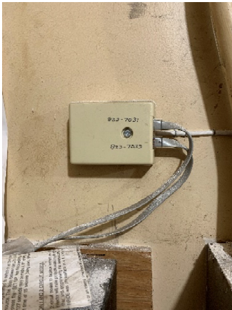
Off-Site Monitoring Lines
