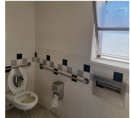
Minor accessibility issues (window protrusion exceeds 4")
