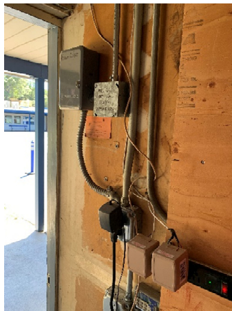
Exterior Lighting Timeclock
