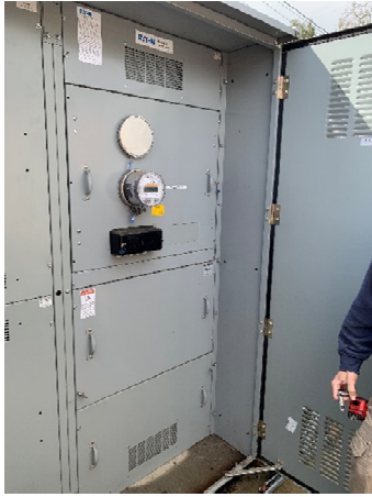
Main Electric Service Panel
