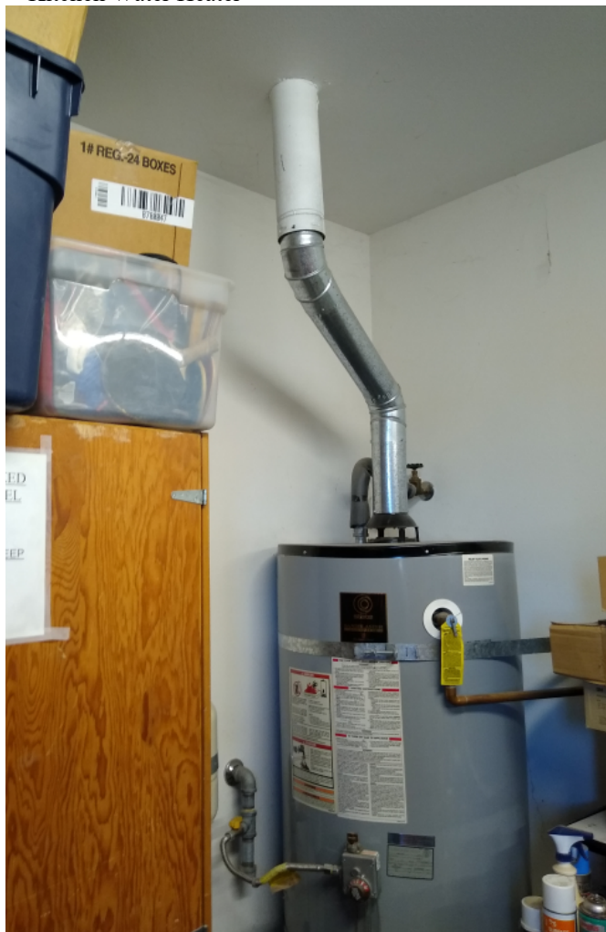
Kitchen Water Heater
