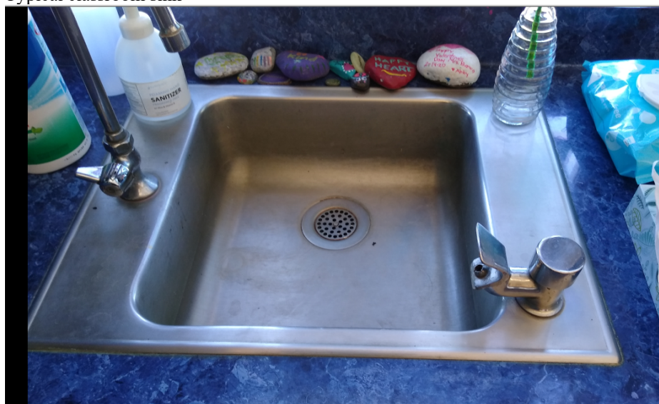
Typical classroom sink
