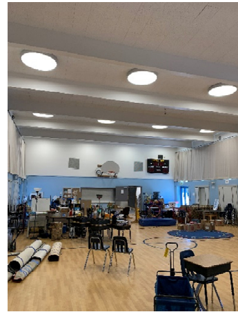
Surface Mtd Lighting
