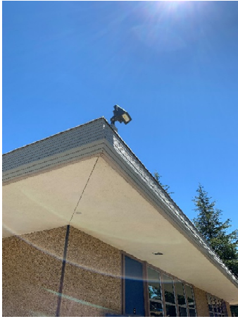
Exterior Roof Edge LED Lighting
