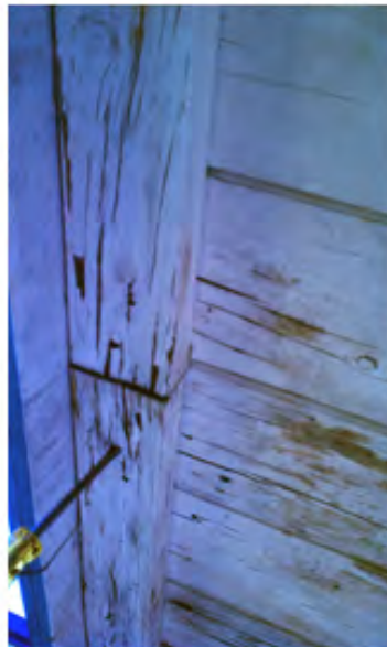
DRY ROT AT SIDING TRIM OBSERVED PRIMARILY AT BUILDINGS C, AND D
