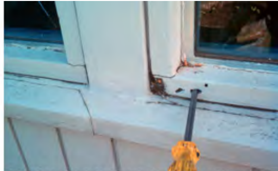
DRY ROT TYPICAL AT EXPOSED WINDOW FRAMES
