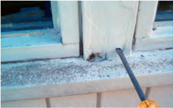
DRY ROT TYPICAL AT WINDOWS EXPOSED TO THE WEATHER
