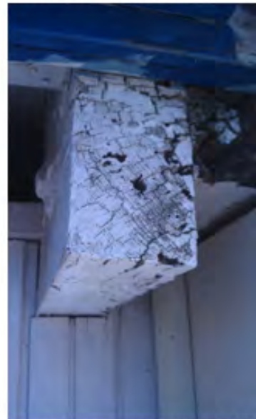
DRY ROTTING ROOF BEAM OBSERVED AT VARIOUS LOCATIONS
