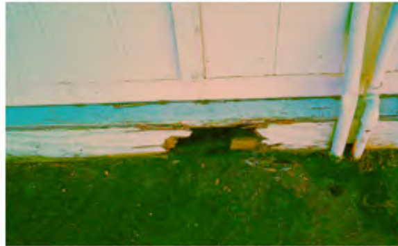
TYPICAL BUILDING FLOOR SILL PLATE IN CONTACT WITH GRADE. THIS WAS OBSERVED PRIMARILY AT THE EAST ENDS OF BUILDINGS A,B AND ADMIN
