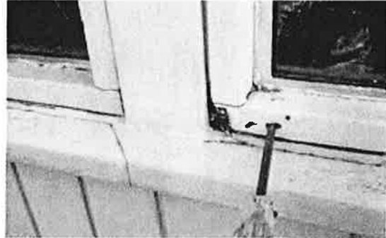
DRY ROT TYPICAL AT EXPOSED WINDOW FRAMES
