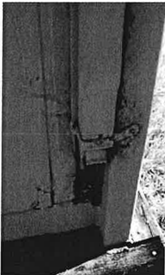
DAMAGED RAIN LEADER AND SURROUNDING FINISH MATERIALS
